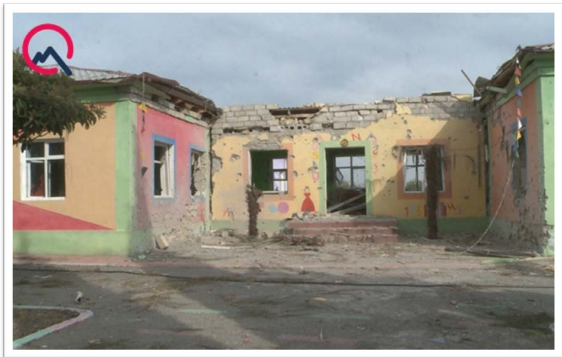
Photo 45-46 (next page) : Kindergarten in the Baharli settlement of the Aghdam district damaged as a result of artillery shelling by the armed forces of Armenia on October 26, 2020
